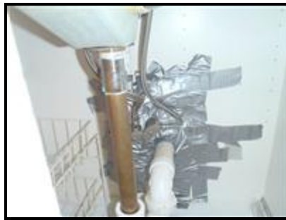
4.1 Picture 1 Large hole under sink vanity with duct tape
