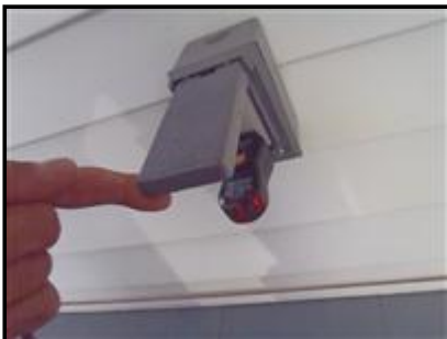
7.4 Picture 1 Front porch GFI was on but did not trip when tested
