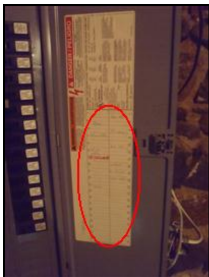
7.4 Picture 7 Not all circuits are labeled
