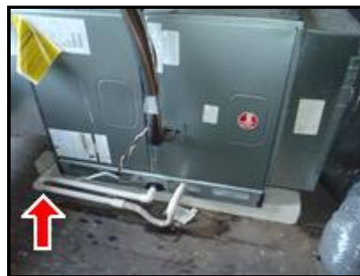
8.5 Picture 1 Condensate lines are teed together and is leaking
