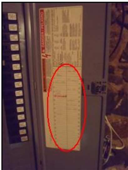
7.4 Picture 7 Not all circuits are labeled
