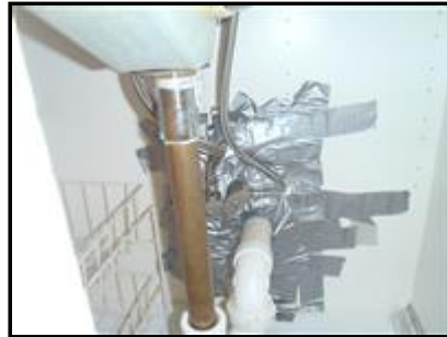
4.1 Picture 1 Large hole under sink vanity with duct tape
