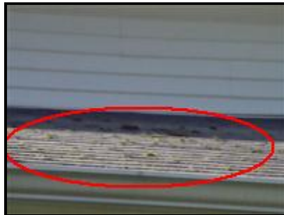
1.0 Picture 1 Moss growing on rear roof shingles
