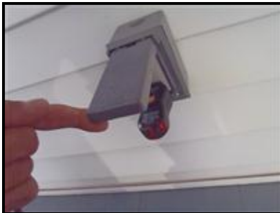
7.4 Picture 1 Front porch GFI was on but did not trip when tested
