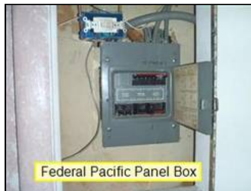
6.2 Picture 1 Federal Pacific panel boxes are
