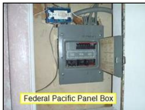
6.2 Picture 1 Federal Pacific panel boxes are fire hazards
